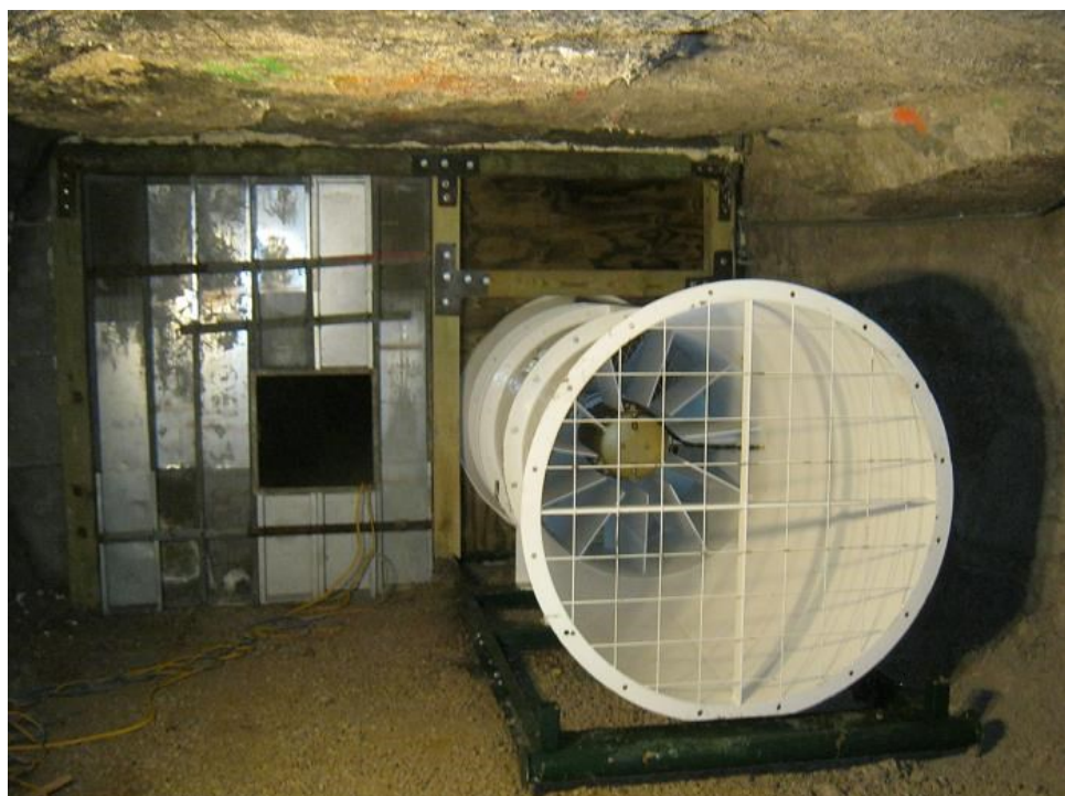
Figure 3.10 Booster fan bulkhead- front view
