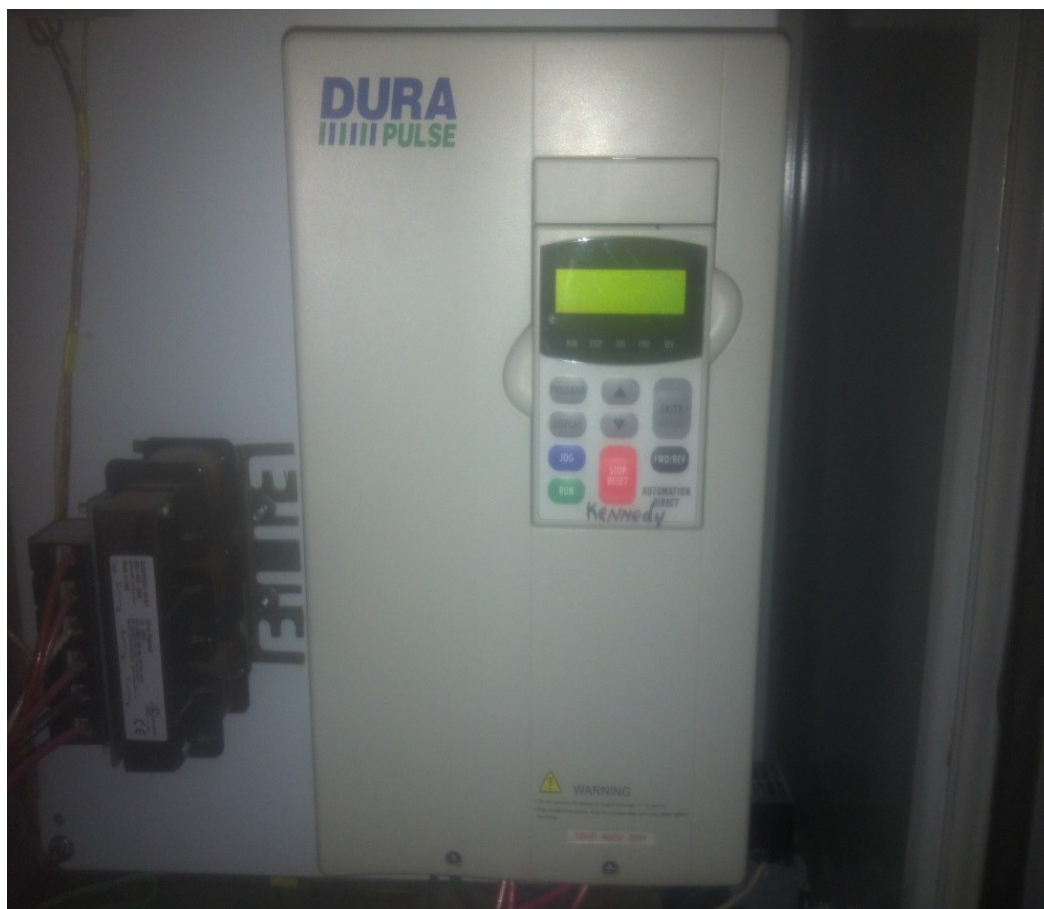
Figure 3.12 Variable frequency drive
